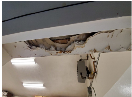
Figure 35: Water damage on ceiling in apparatus bays
